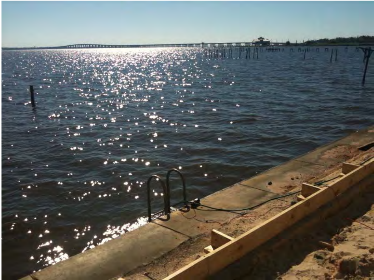
Figure E3B.2 Photographs of Bay Saint Louis
