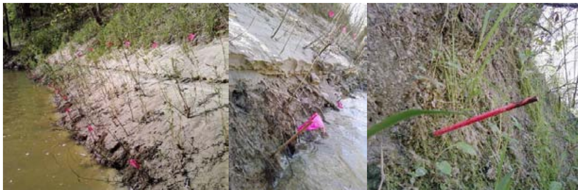
Figure 22. Pin erosion plots to determine streambank erosion rates at Town Creek, MS
